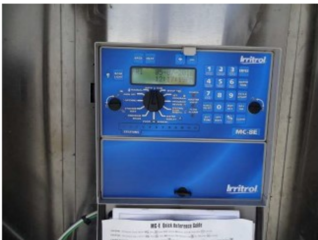
Figure 15.5: Irrigation System Selector Switch.
