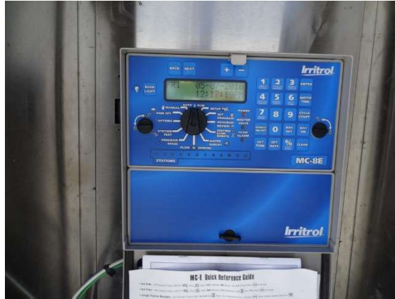
Figure 15.5: Irrigation System Selector Switch.
