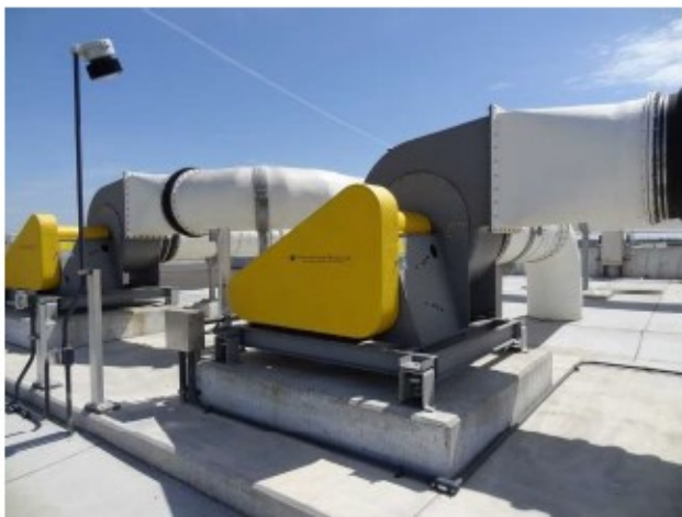
Figure 15.2: Foul Air Supply Fans.
