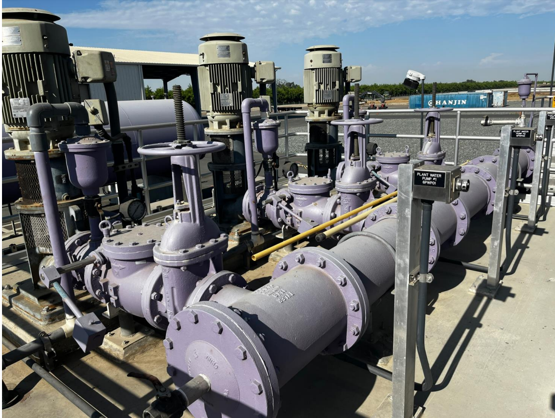
Figure 14 Plant Water Pumps
