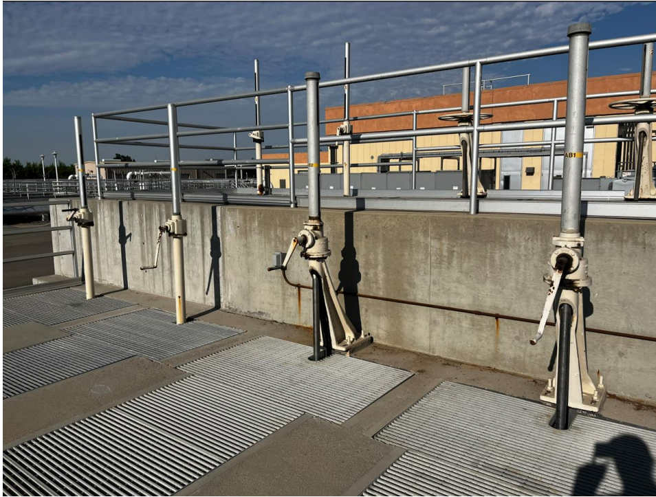
Figure 7 Junction Box A
