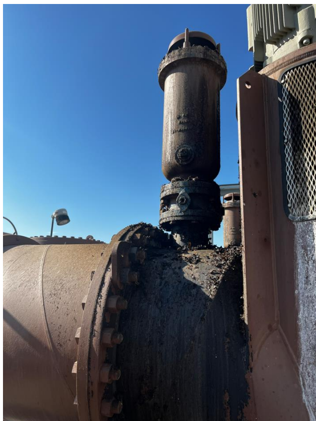
Figure 12 RAS Pump – Sludge Spillage
