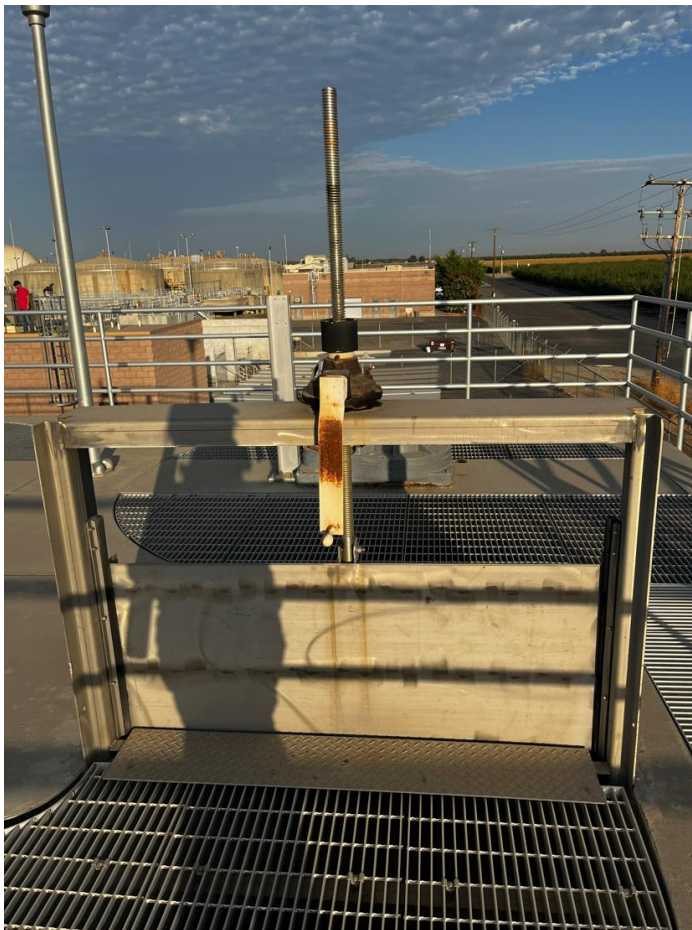
Figure 1 Gates in Grit Basins – Corroded Hand Crank
