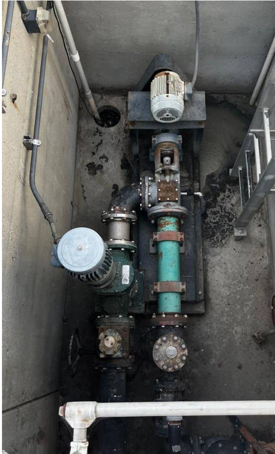
Figure 5 Scum Box No. 1 – Corrosion on Piping
