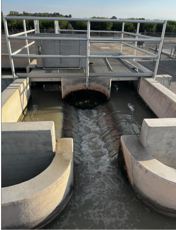
Figure 4 Primary Distribution Box B
