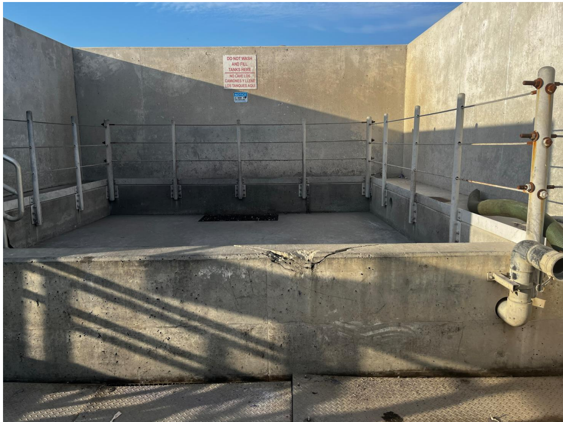
Figure 2 Septage Receiving Station – Cracked Concrete
