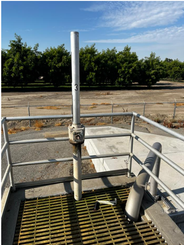
Figure 8 Corrosion on Gearbox
