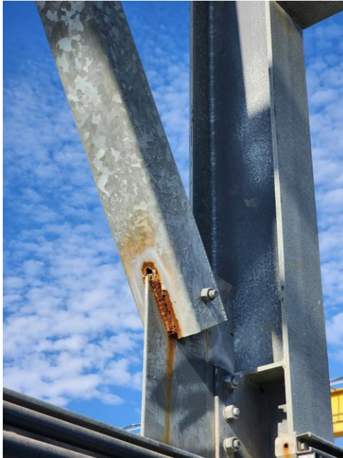
Figure 9 Braced Frame near MBR -Corrosion at Brace and Gusset Connection
