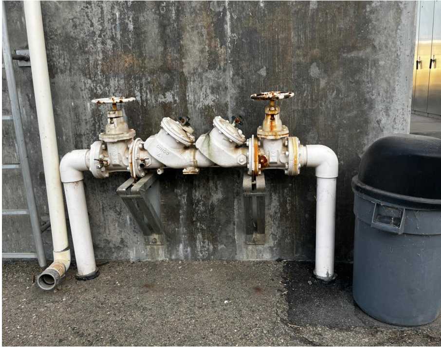
Figure 3 Piping by the Flow Split Structure
