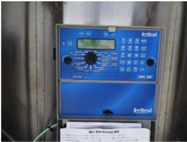
Figure 15.5: Irrigation System Selector Switch.
