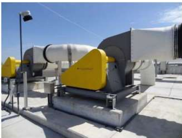
Figure 15.2: Foul Air Supply Fans.
