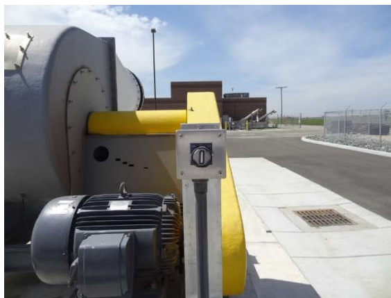
Figure 15.4: Biofilter Fan HOA Selector Switch.
