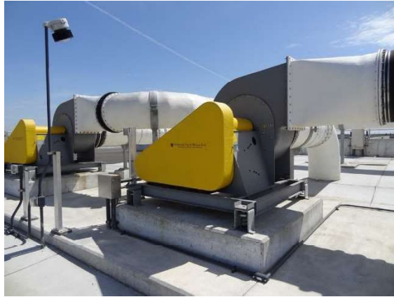
Figure 15.2: Foul Air Supply Fans.
