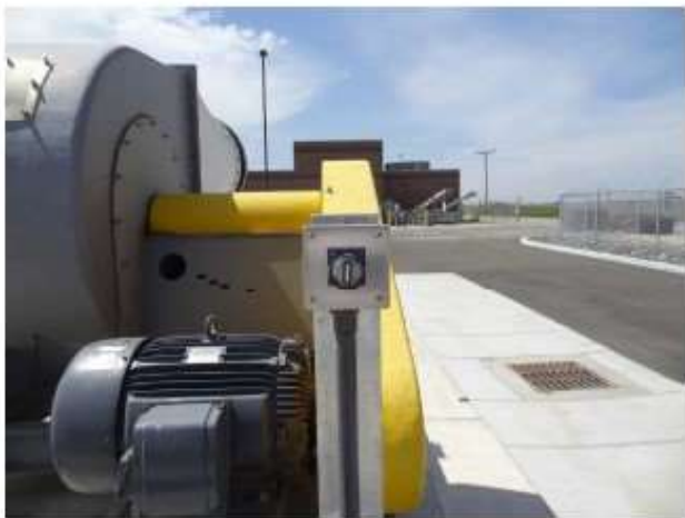
Figure 15.4: Biofilter Fan HOA Selector Switch.
