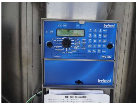
Figure 15.5: Irrigation System Selector Switch.
