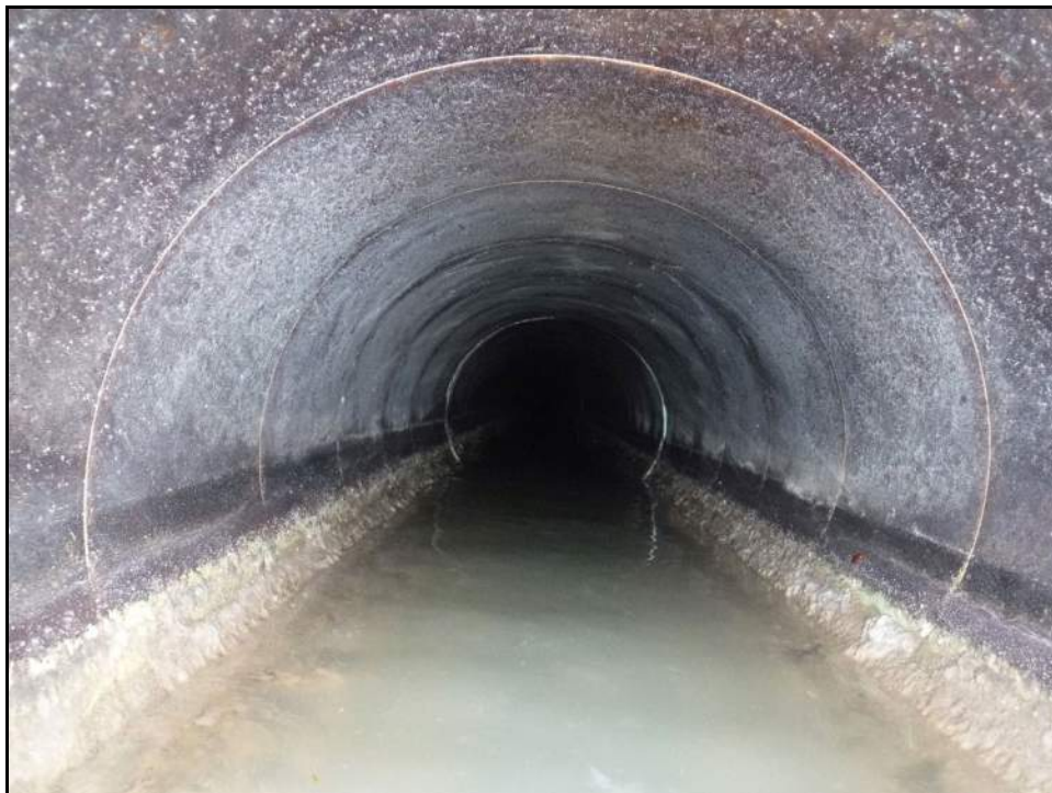
East Influent Pipe
