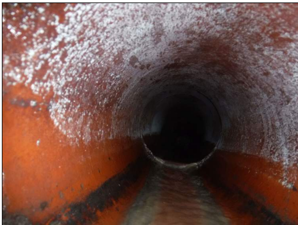
East influent Pipe
