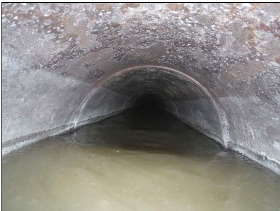
North Influent Pipe
