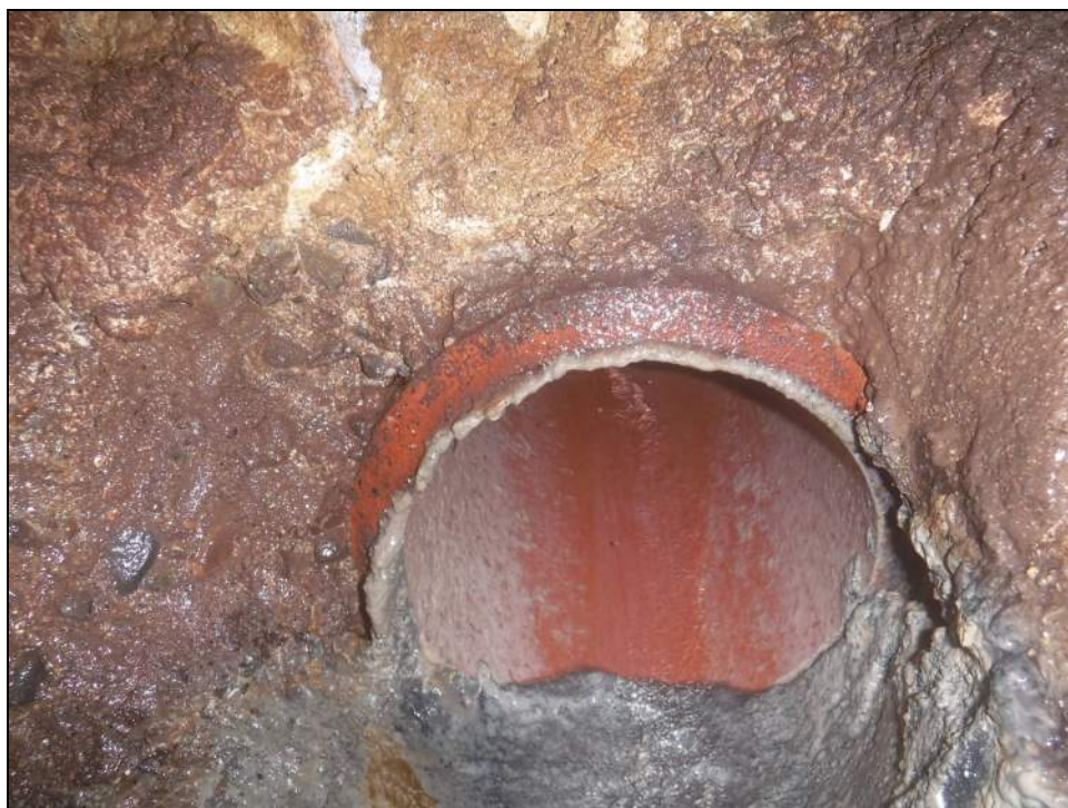
North Influent Pipe
