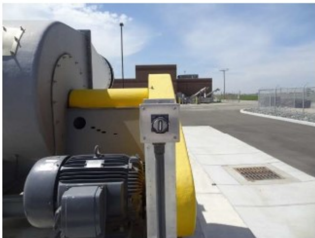
Figure 15.4: Biofilter Fan HOA Selector Switch.
