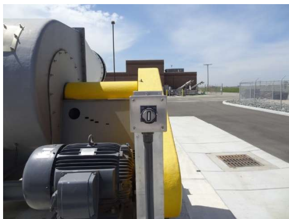
Figure 15.4: Biofilter Fan HOA Selector Switch.
