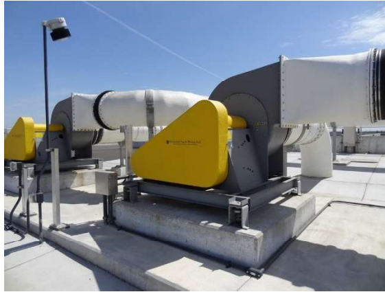
Figure 15.2: Foul Air Supply Fans.
