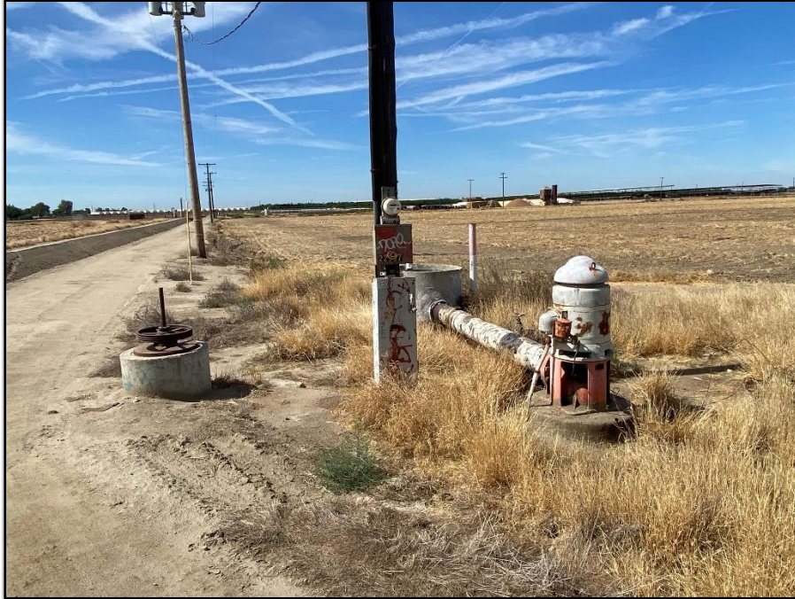
Figure 4-7 Water pump on the Project site, facing south.
