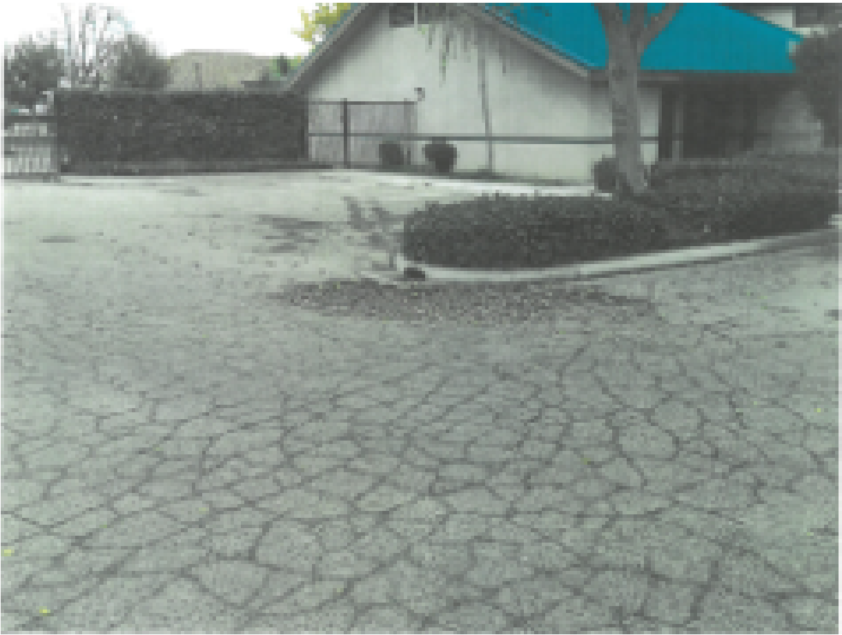
FIGURE 1 - PAVEMENT FAILURE - DIGOUT AND STRUCTURAL CONCRETE REQUIRED
