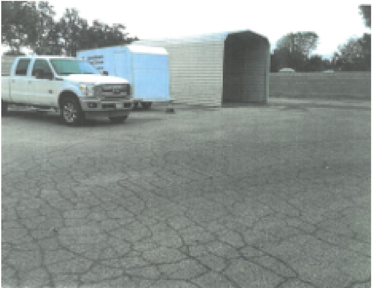
FIGURE 2 - SURFACE CRACKING - MICROSURFACING TREATMENT
